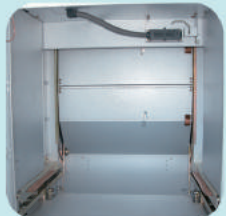
Circuit breaker compartment of AMS-40.5kV
