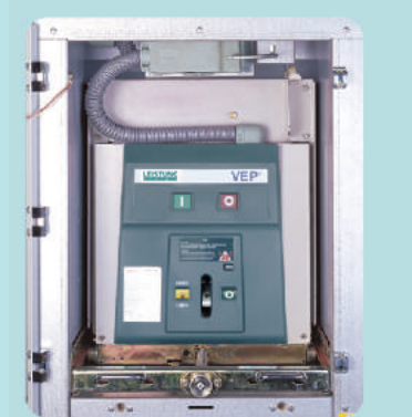
Circuit breaker compartment of AMS-12kV
